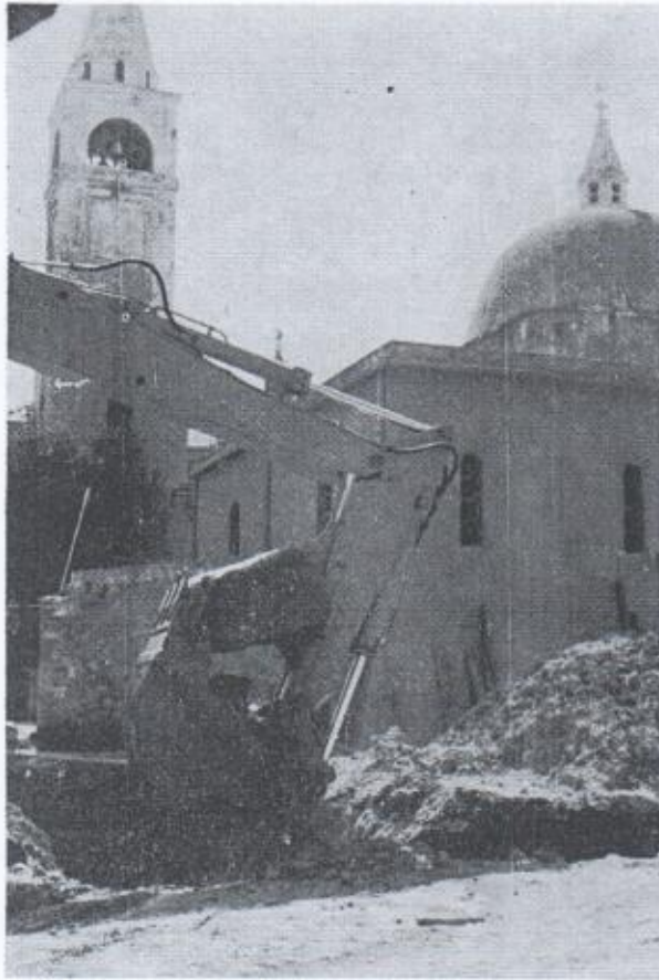
The rear of the church of S. Maria in 1975 during the work which uncovered the ancient church in the new part of the city.
